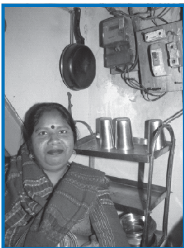
Electricity meters installed
